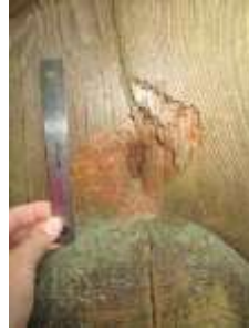
Example of damage caused by the feeding activities of the woodpecker.
